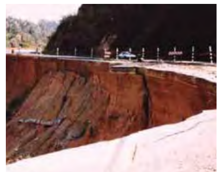
Figure 5.3: Some areas are prone to landslides
