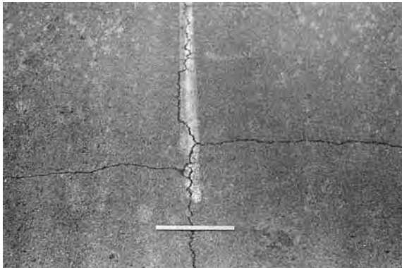
Cracking outside wheeltracks – block cracks
