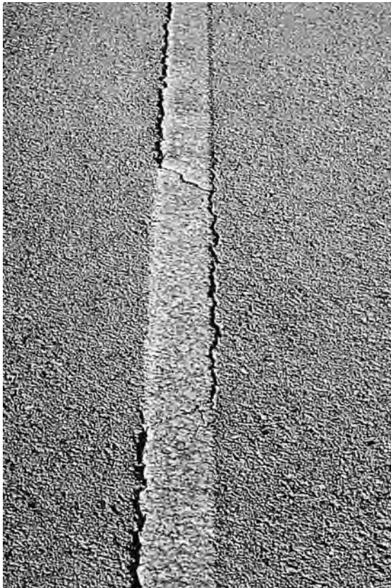
Cracking outside wheeltracks – along white line
