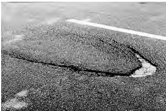
Cracking outside wheeltracks – parabolic crack
