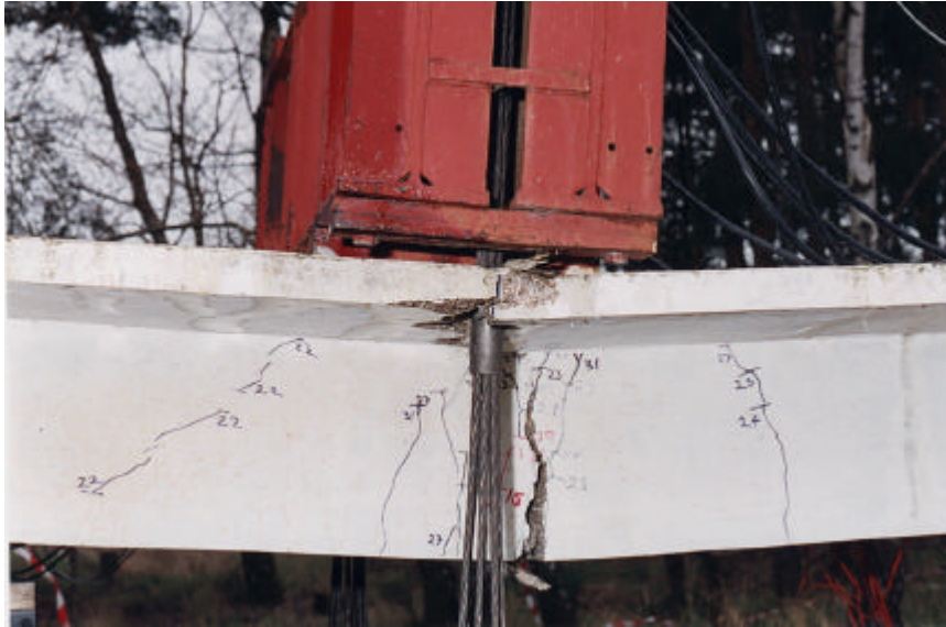
Figure 9 Failed model after load test 2.
