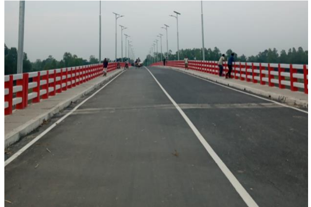
g) Wide bridge expansion joints will create passenger discomfort
