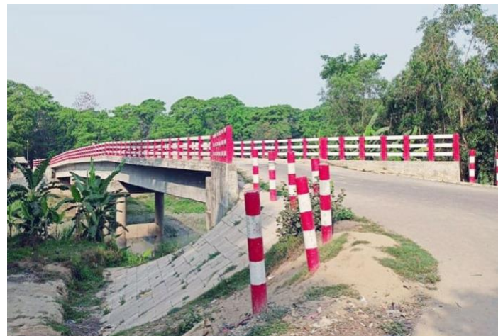
d) Steep approach road may result lack of control; also notice the gap between edge barrier posts and sharp turn
