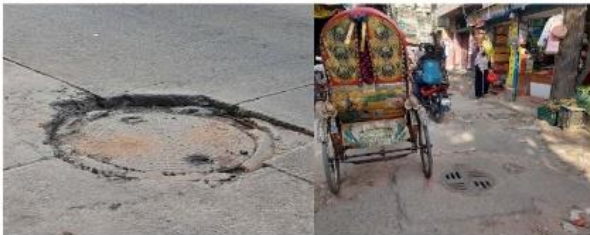
5. Uneven manhole cover/pit slab
