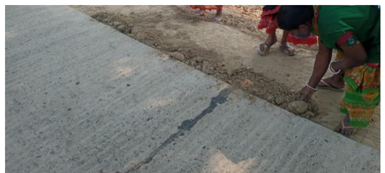
d) Expansion joints as well as rigid pavement texture may result discomfort for Tri-SMV users while steep shoulder drop may result accidents
