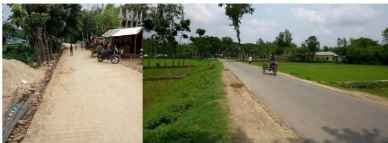
7. Insufficient Shoulder Width/Pavement Edge Drop-off
