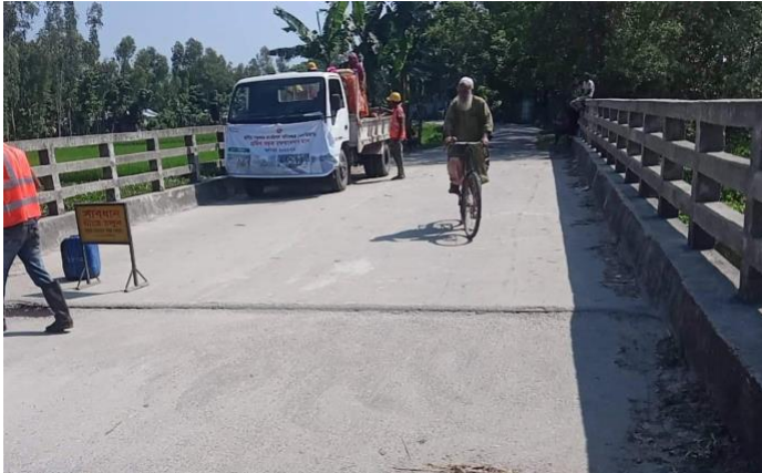
f) Vertical gap between bridge approach and bridge deck will create significant distress for Tri-SMV users
